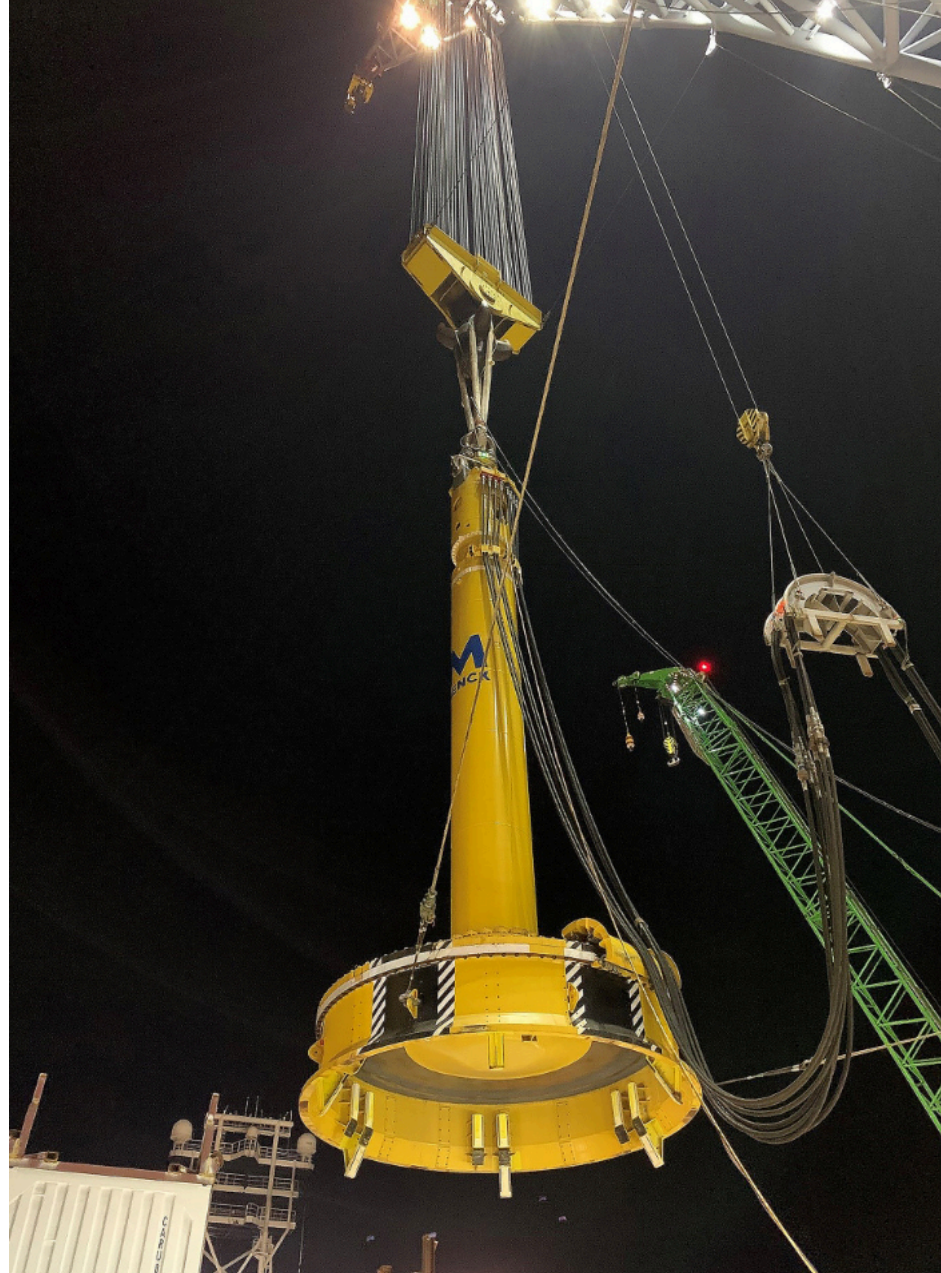
A MENCK hammer being utilised on Vattenfall's Hollandse Kust Zuid I-IV (HKZ) offshore wind farm project in the Netherlands'
