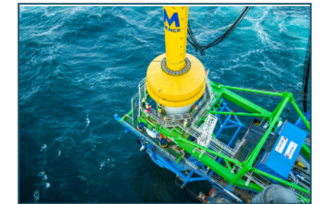
A MENCK hammer being utilised on Vatten fall's Hollandse Kust Zuid I-IV (HKZ) offshore wind farm project in the Netherlands'
