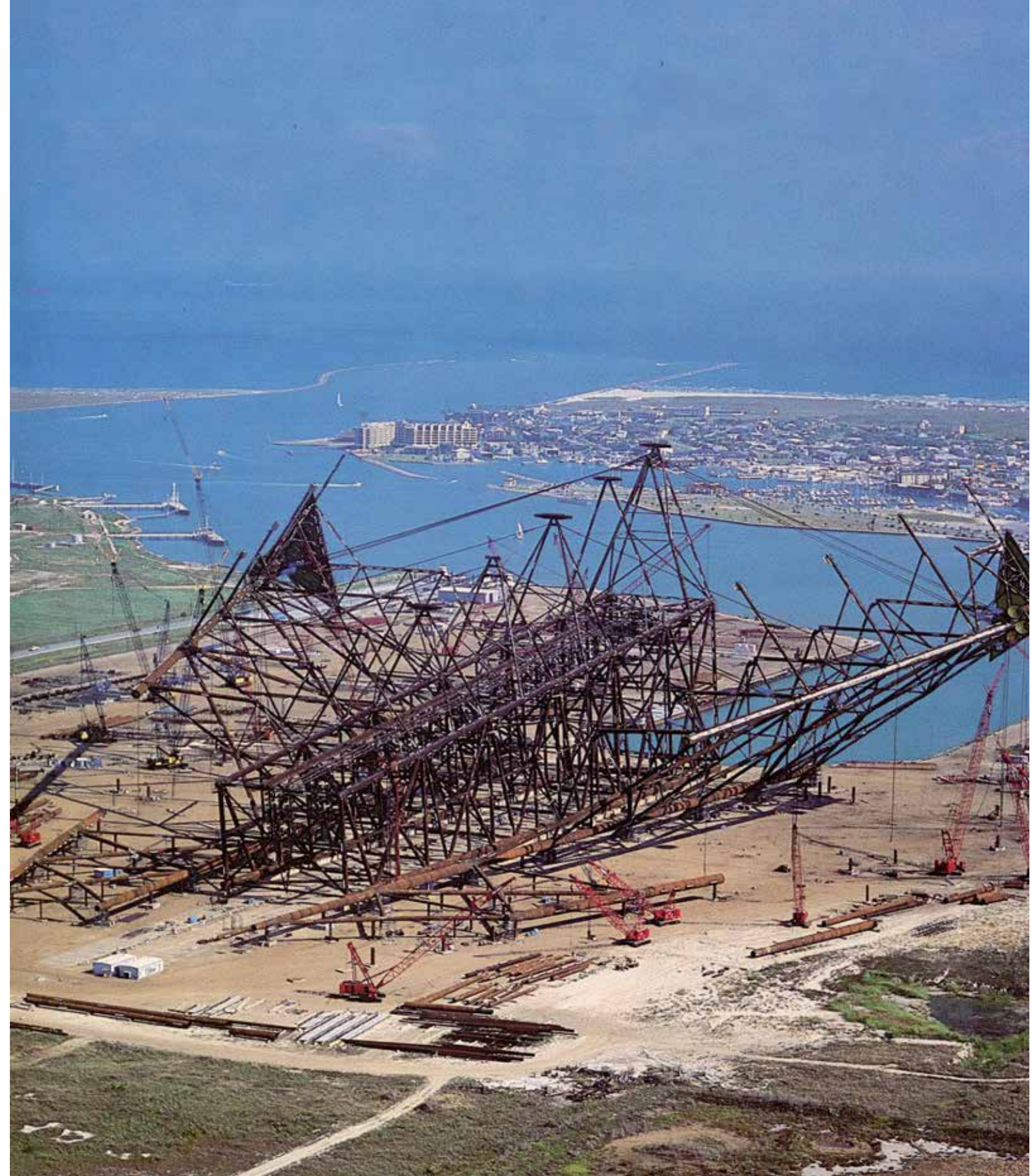
The Harbour Island fabrication site. Work begins on the roll-up of the 6500t outer panels of BP's Pompano Jacket.
